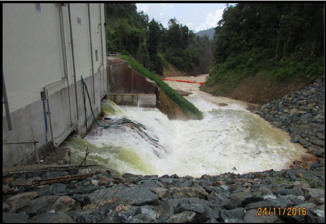
Tembat Tailrace and Boat boom – Turbine output at 105% rated flow (~ 14 m 3 /s)
