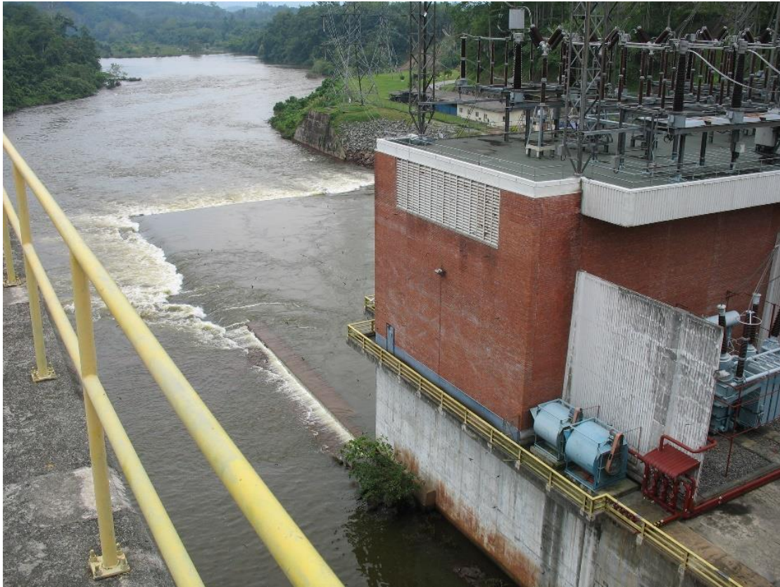
Bersia powerhouse 2006; tailwater weir, switchyard on the roof
