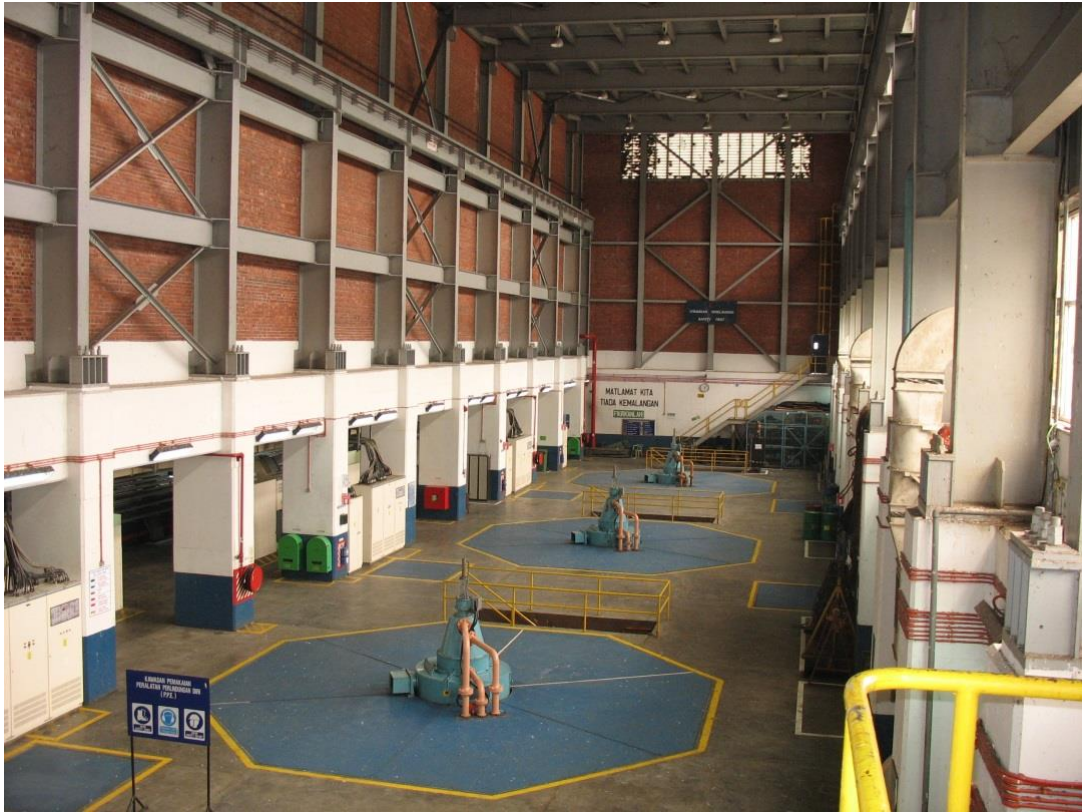
Bersia Powerstation interior 2006
