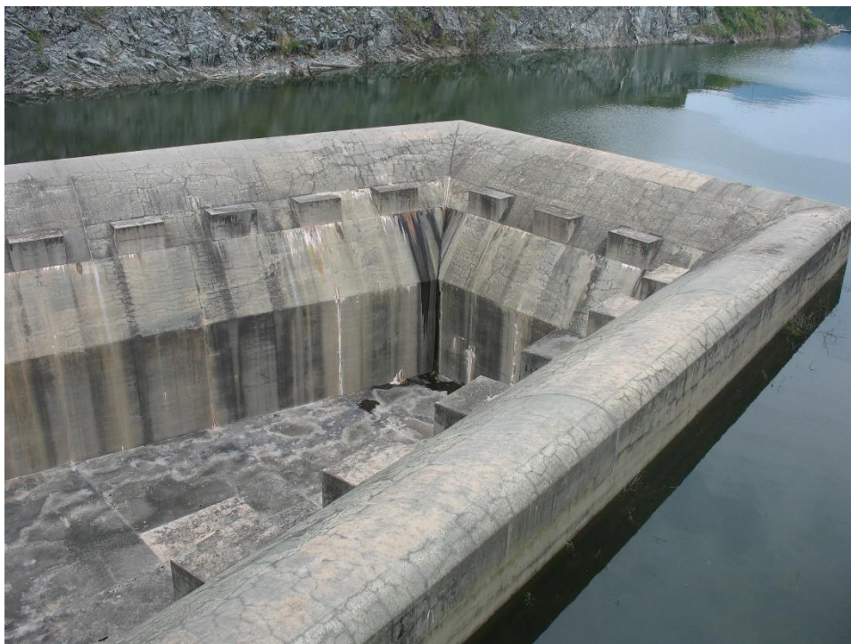
Overflow spillway. Heavily crazed probably due to finishing technique! (2006 Photo) (Note: the 2004 Dam safety Report stated the cracking might be due to AAR.)
