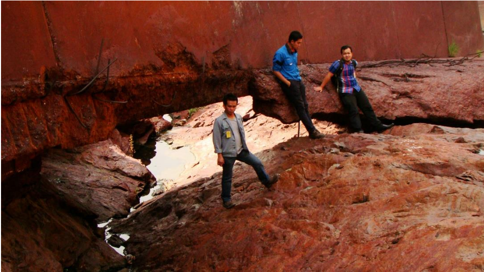
Wash-out below left side wall inside view.
