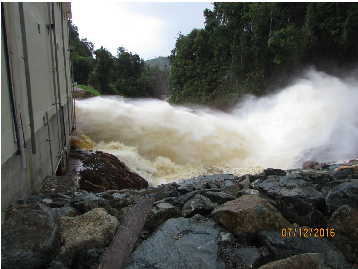
Tembat Hollow cone valve operating at about 15 m 3 /s
