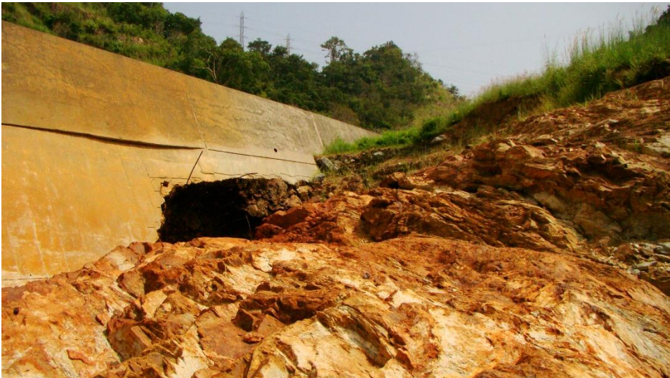
Wash-out below left side wall outside view.
