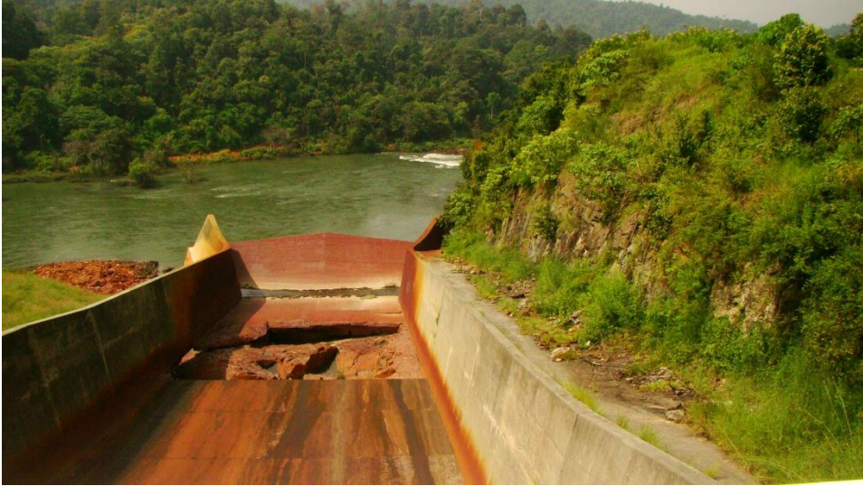
Washed out slab.
