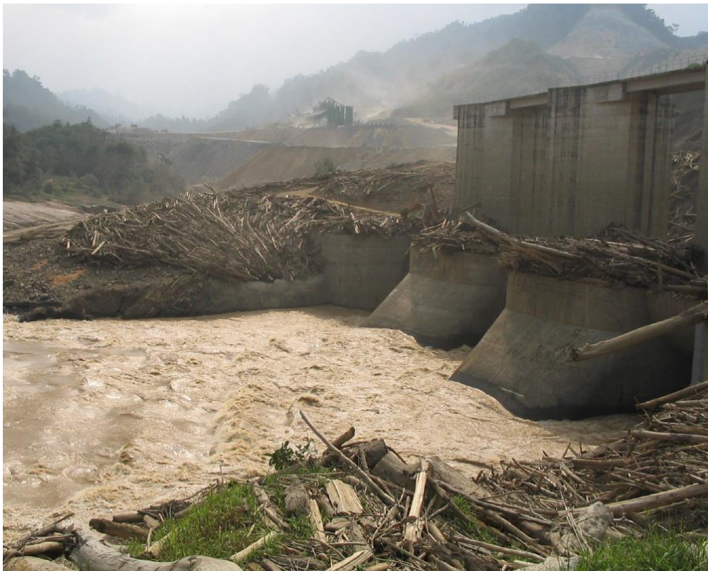
Intake to 3 No. x 13m dia. Diversion Tunnels. Post impounding it was reported that 250,000 tonnes of driftwood were trapped by the Worthington log boom.
