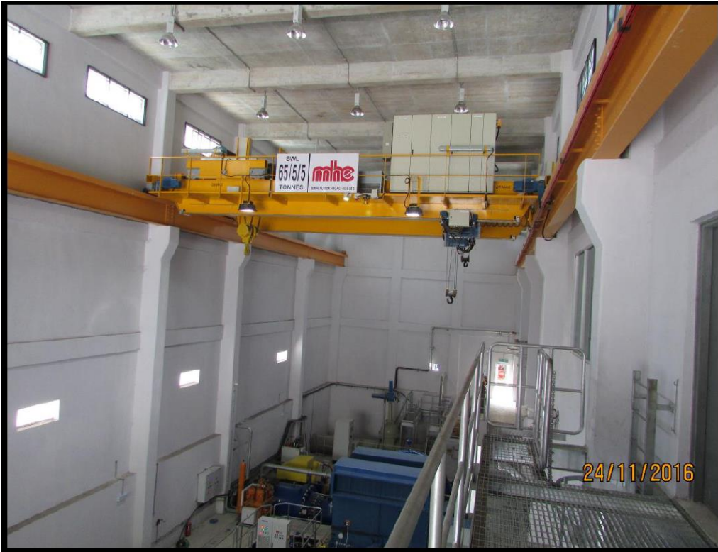
Tembat Powerhouse – 65 tonne EOT Crane
