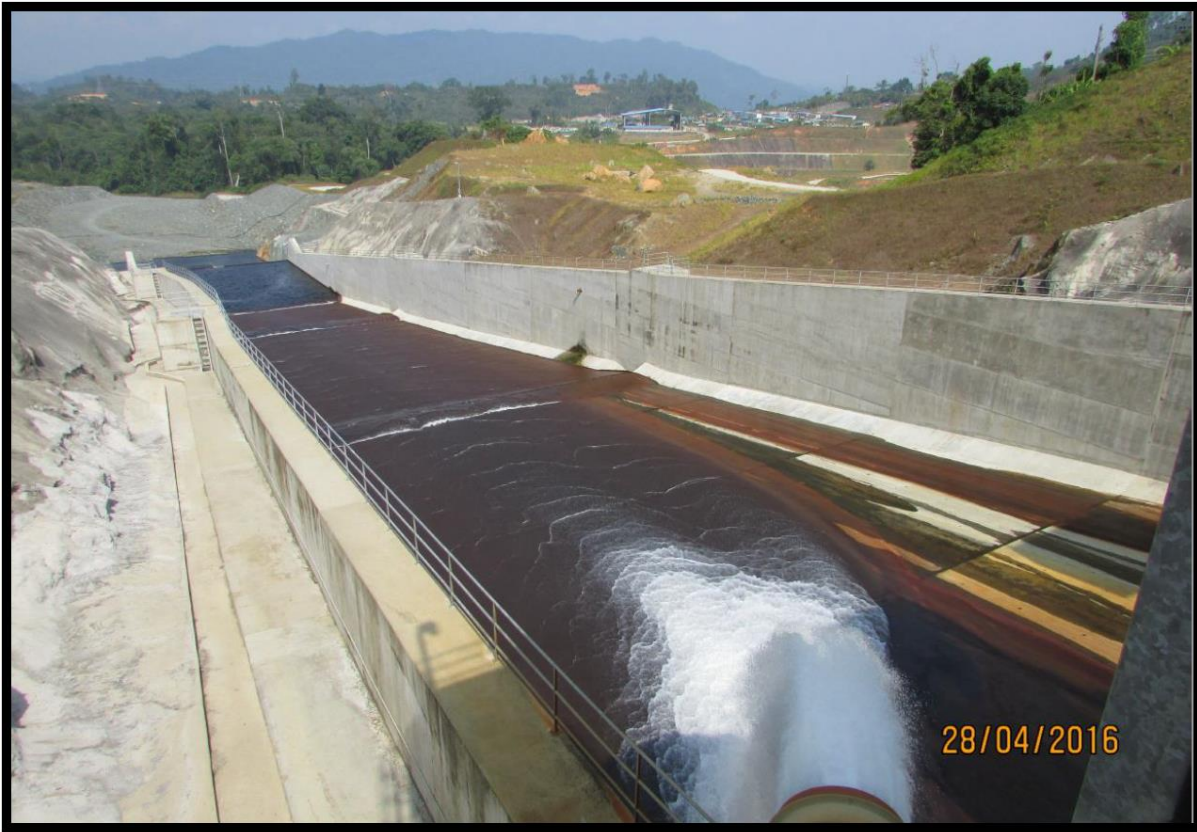
Puah Spillway with Riparian release flow of 1.0 m 3 /s
