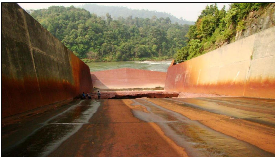
Failed slab section
