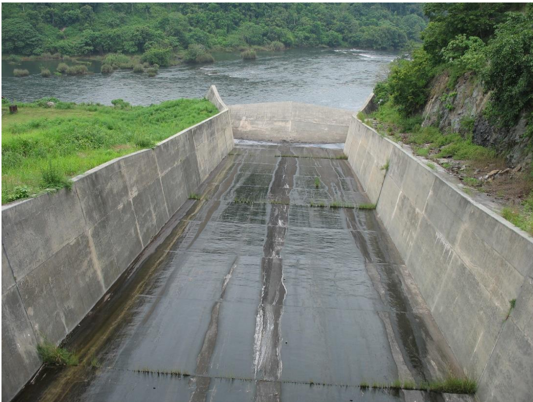
Lower section of chute where failure occurred viewed from Bridge. (photo May 2006)
