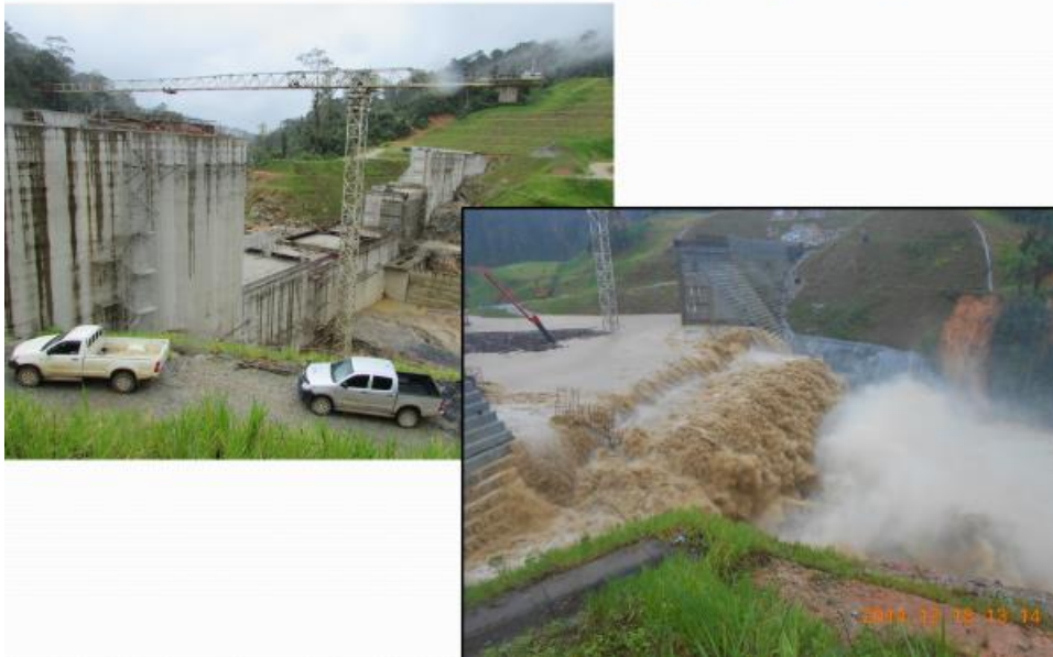
Tembat dam overtopped by monsoon flood during construction
